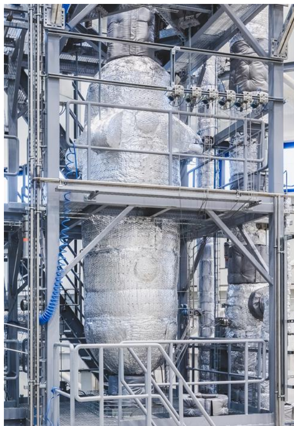
Figure 2-3: Primary heat exchanger of S-Allegro facility (installed)
